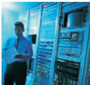
Servers, data storage and network equipment
